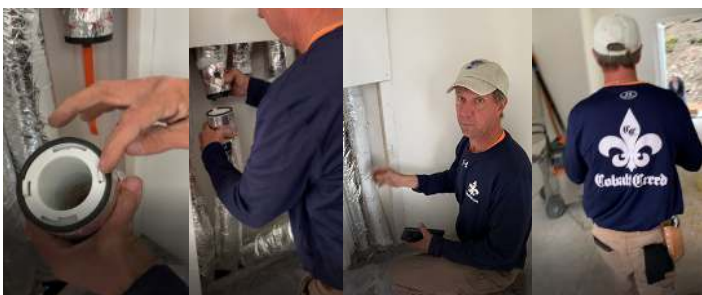
Mickey Lubinski, Cobalt Creed Engineer, MODULE home-site location: installation of the Unico Twist-Fit System™
